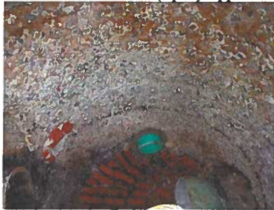
Hydrogen Sulfide Erosions
