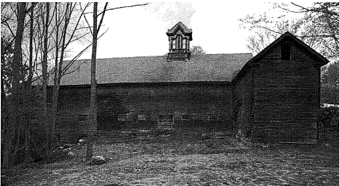
Figure 6. South elevation with silo ell at right. Photograph by John Butler. (May 15, 2003)
