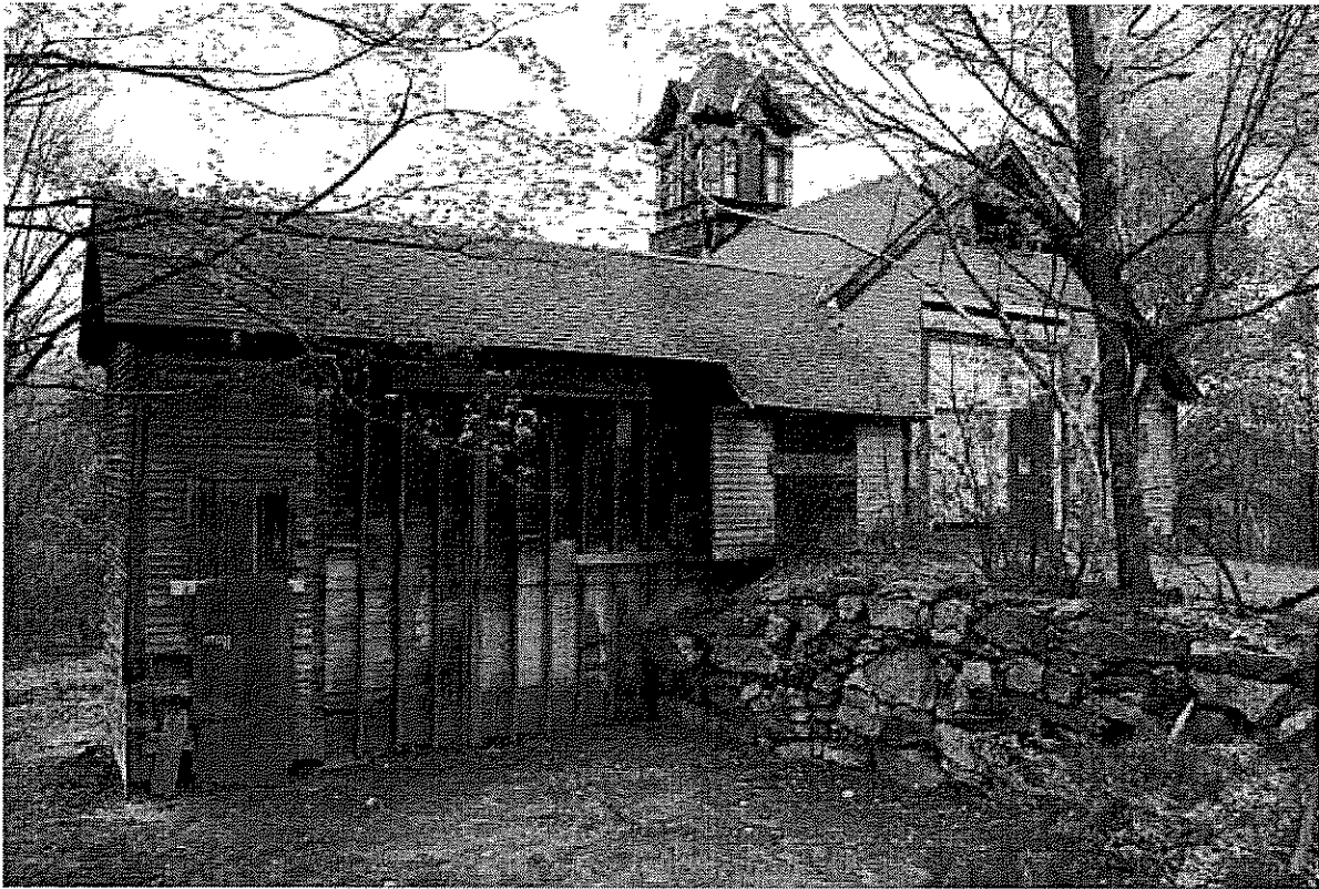
Figure 4. East (front) elevation with granary ell in left foreground. Photograph by John Butler. (May 15, 2003).
